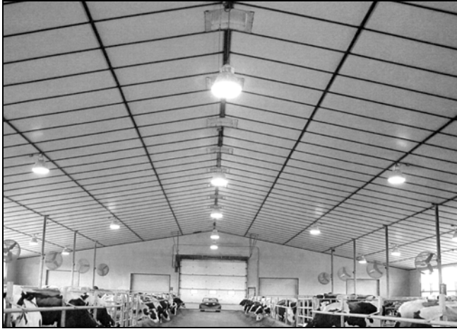
FIGURE 7. Metal halide fixtures.
